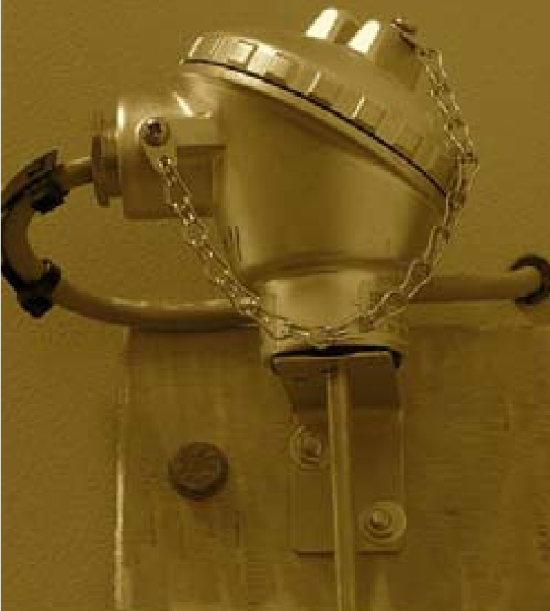
VALVE ROOM TEMP. TCR-3. BTB.4
